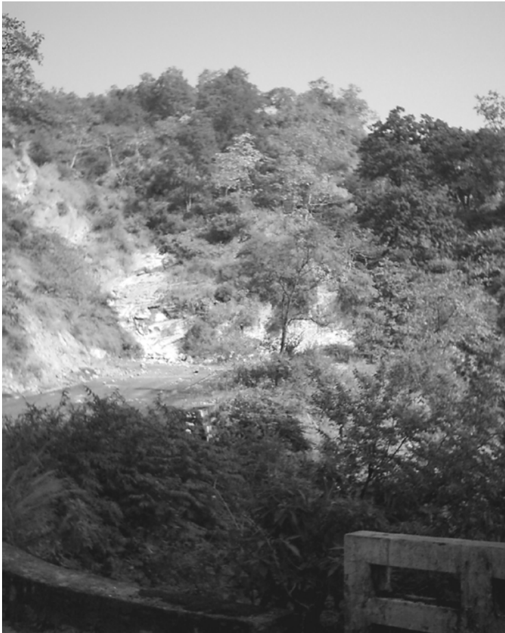
Plate 2 Road Damaged by Mansa Devi Landslide
