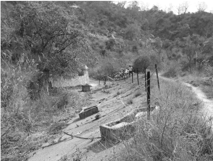
Plate 1 Slided Soil Mass had Tilted the Road
