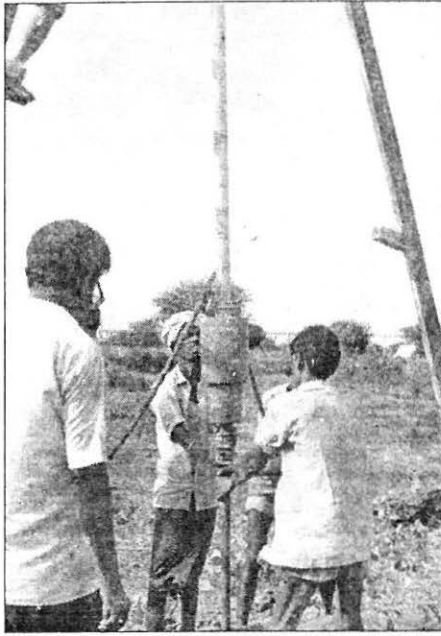
FIGURE 2 : Crude Method, No Safety Measures, No Assurance of Vertical Application of Load
