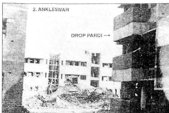
FIGURE 43 : After Collapse of Structure
