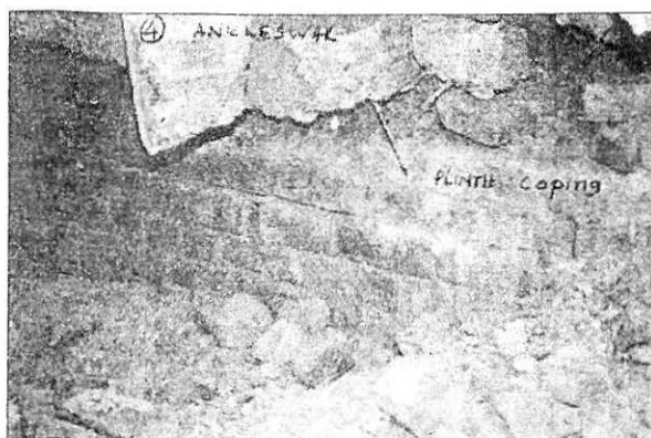
FIGURE 45 : Wall below Plinth after Collapse
