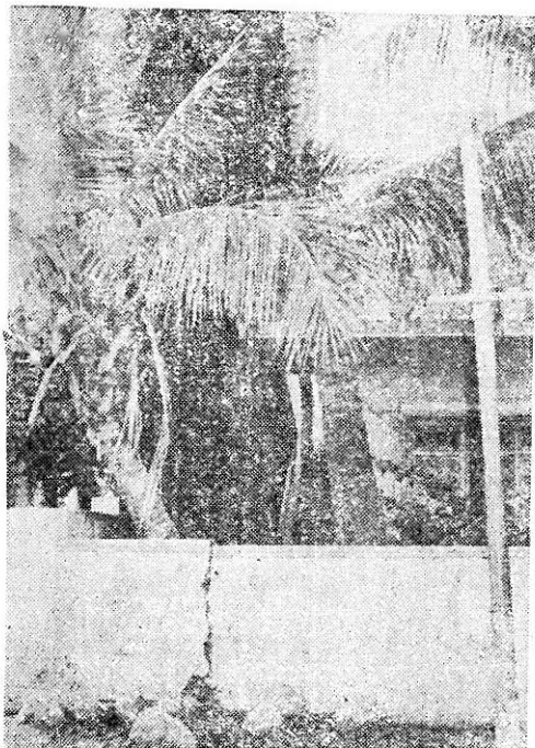
FIGURE 9 Cracking at A
