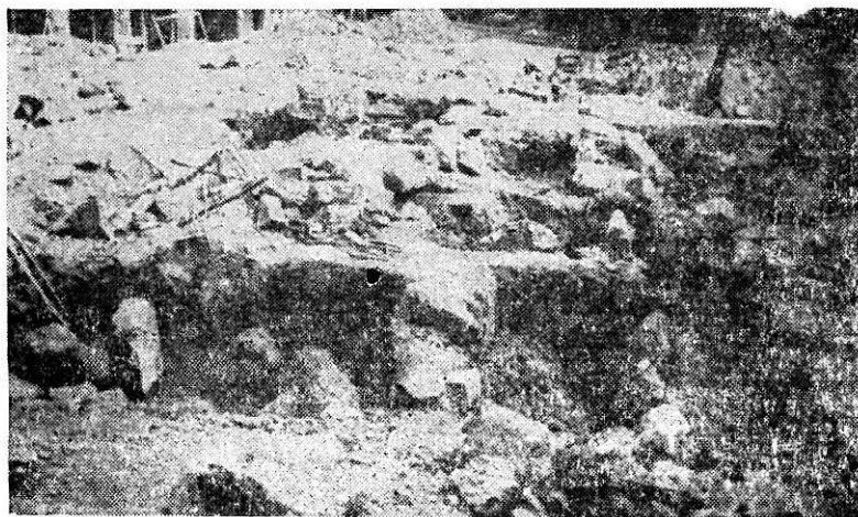
FIGURE 11 View of the North-West Column which Punched First through Pile Cap and Piles and Adjoining Drain Beneath the Building.
