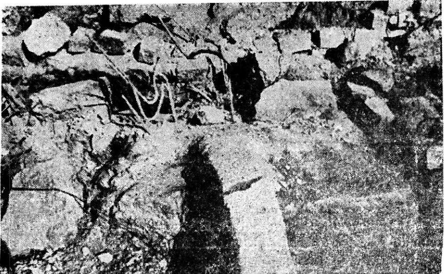
FIGURE 13 Cracking of Pile Cap Connecting Beam Supporting Office Wall which Crumbled First.
