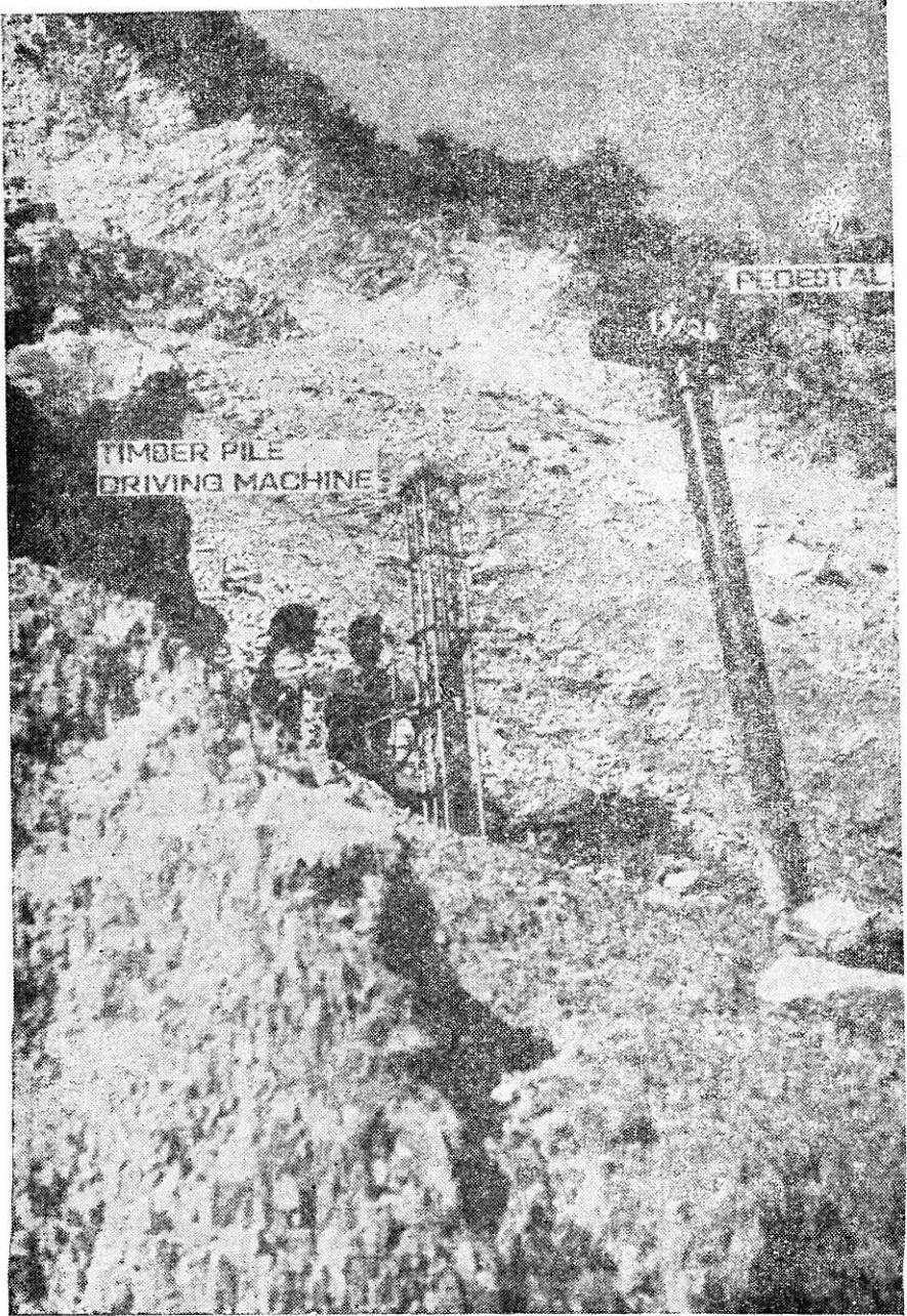
FIGURE 27 Stitch of Colluvium on the Slope at Kaliasaur by a Simple Lowcost Timber Piling Machine
