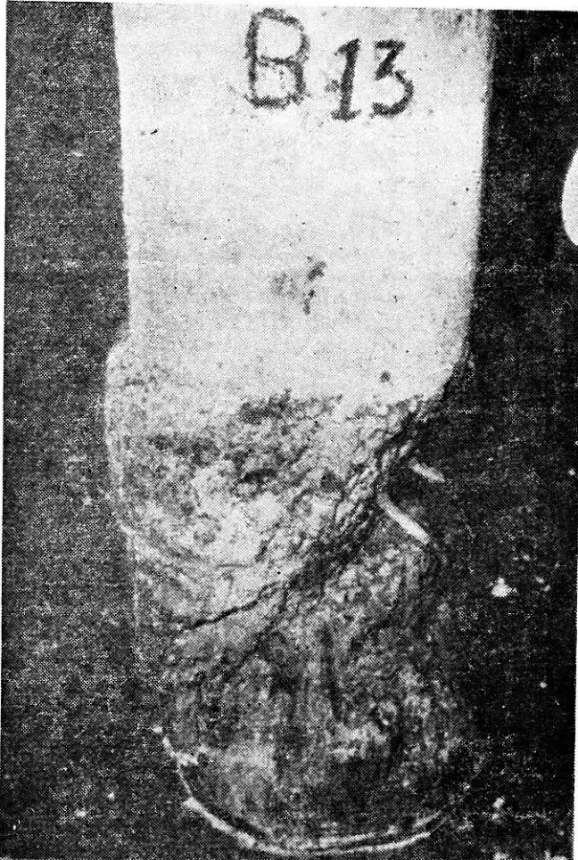
FIGURE 8 Typical illustration of defective driven cast in-situ pile
